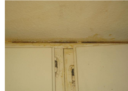
Gaps between Kitchen Cabinets
