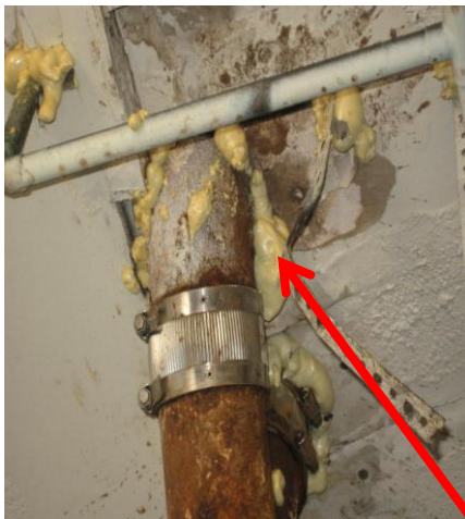
External Water Pipes- Damaged and corroded
