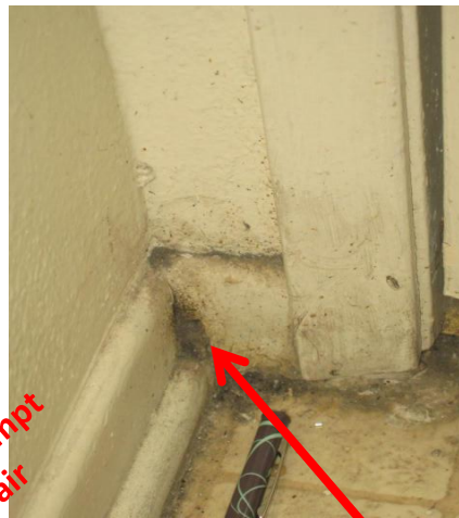
Cracks and Crevices- Hiding places for roaches
